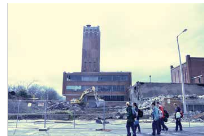
As a part of the UTHSC Campus Master Plan, the Beale Building was demolished in April to make way for new developments.
